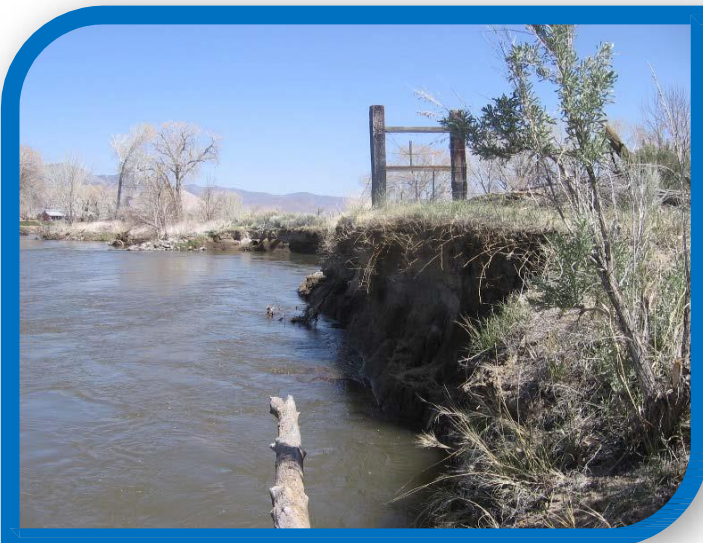
Flooding at Minor Ranch, 2017, showing extent of bank erosion
